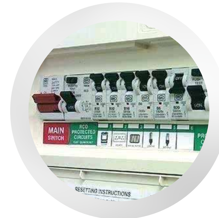
Circuit Breakers Appliances, Outlets & Lights
